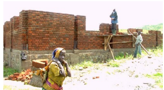
The Baraka Baptist Church is being built with funds from the Swahili Baptist Church and Woodmont Baptist Church, Nashville.
